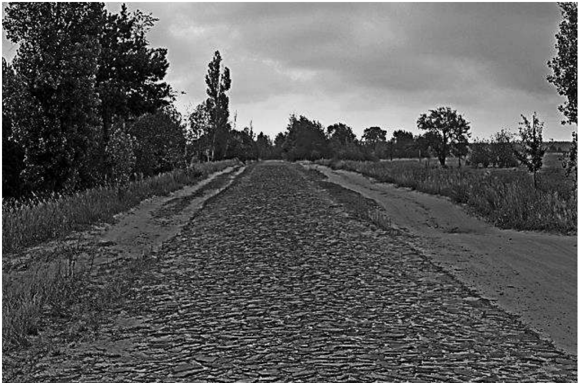
Fig. 8. Reconstruction of a dirt road in a road with a solid pavement
