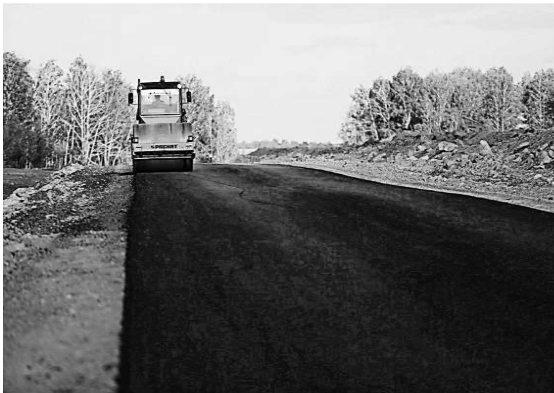
Fig. 10. Inherited negative engineering-geodetic, structural and operational features of the dirt road during reconstruction of the highway
